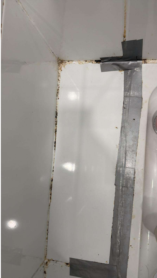
PHOTO 01: The photograph shows a bathroom or wet room corner with extensive black mould growth along tile grout joints and panel edges, combined with heavily deteriorated and failed grout/sealant. Duct tape has been applied as a makeshift repair to the panel joint, indicating a known water ingress or movement issue that has not been properly addressed. The mould coverage across multiple grout lines and the corner junction is substantial, likely exceeding 0.25 m 2 , and represents a significant health hazard under HHSRS. The improvised repair with duct tape is not a compliant or durable waterproofing solution and will be contributing to ongoing moisture ingress.
